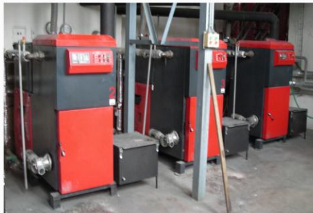
Health center Broumov Cascade of automatic boilers VERNER
