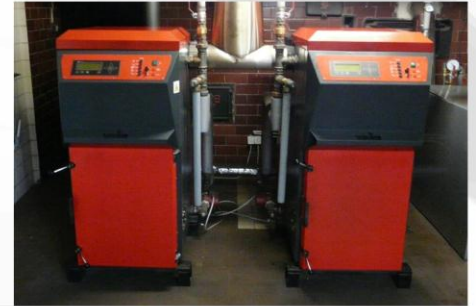
Hotel Tanečnice Pustevny Cascade of automatic boilers VERNER
