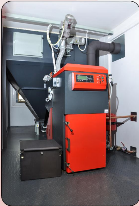
Up: view in mobile boiler room.
