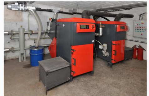
Municipal office and sports hall Vlčice Cascade of automatic boilers VERNER
