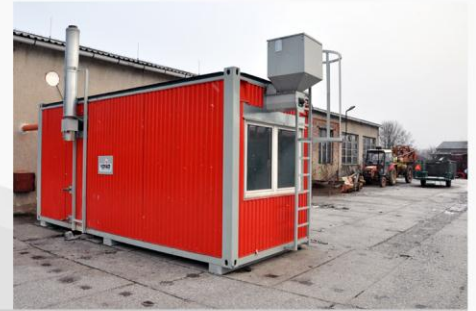
Collective farm Unčovice Mobile boiler room 50 kW
